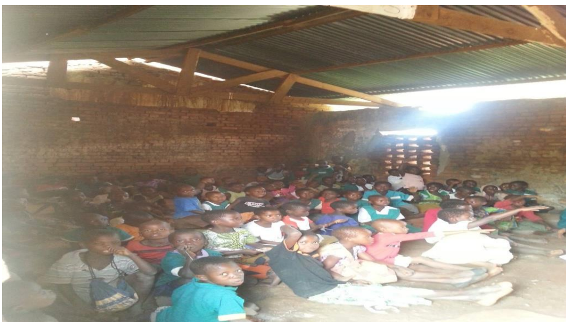
d. Dilapidated classroom in use (source: In-depth study 2016)
