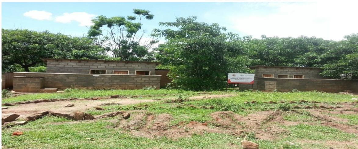
a. Improved latrine with a hand washing facility in front (Source: In-depth study 2016)
